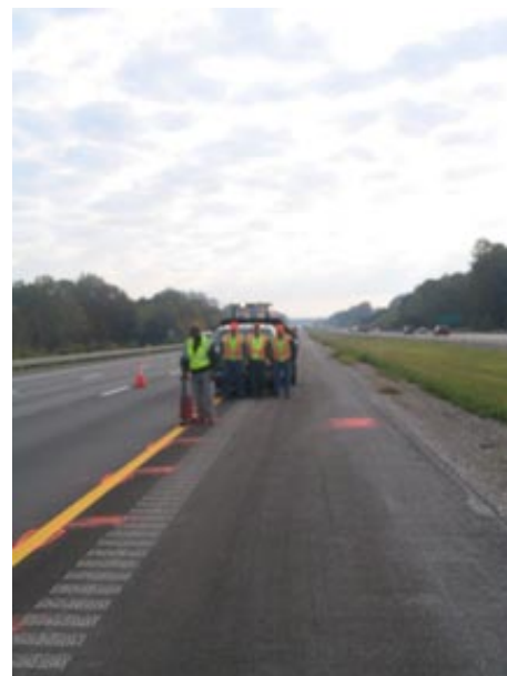
Godswill Nsofor takes measurements on Interstate 40 with the assistance of Tom Talbert, Rick Johnson and Marshall Anderson from TDOT's Region 1 Headquarters.
