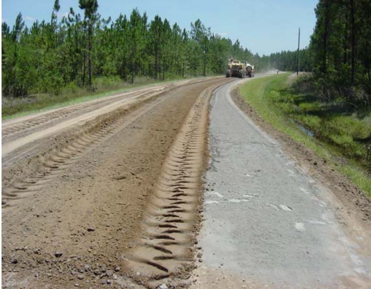
FDR with cement recycles existing asphalt pavements and aggregate bases to create a thicker pavement structure and a longer lasting base.
