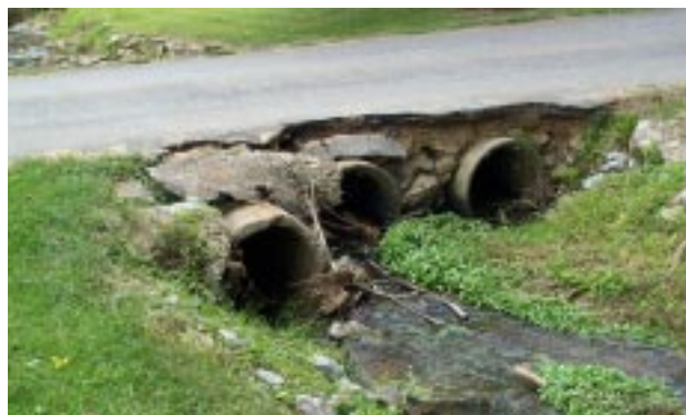
A headwall structure may have prevented the soil erosion and subsequent loss of pavement structure pictured at this three-barrel precast concrete culvert.
