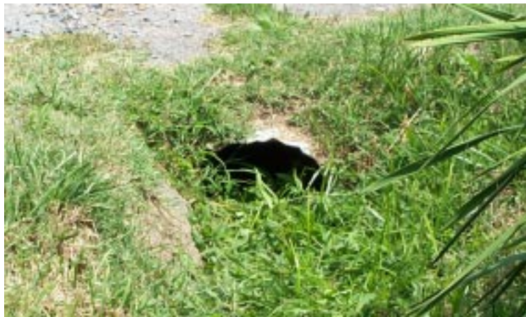
This corrugated metal culvert displays a significant loss of capacity due to excessive sedimentation both in the culvert itself and in the ditch leading to the culvert inlet.
