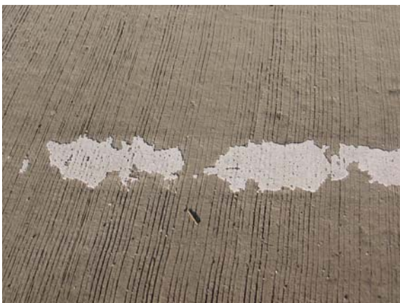
A close-up of the same line shows that as much as half of the original area of the marking has been lost, reducing the available amount of retroreflective material by the same amount.
