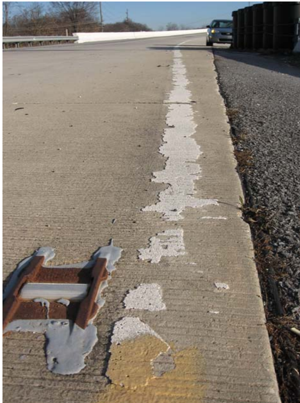
The freeway off-ramp edgeline pictured above is clearly showing the effects of years of damage caused by traffic, weather, and plowing.
