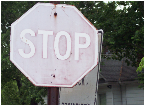
Some signs, such as this badly worn stop sign, require little more than a brief visual inspection to determine that they will not meet new sign retroreflectivity standards.
